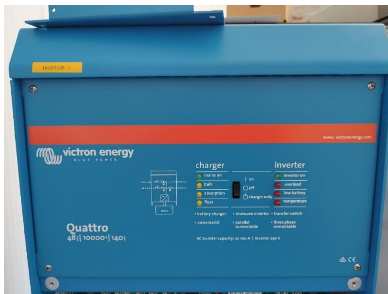
Figura 29 - Painel Principal do Inversor Carregador Quattro 48/10000/140-100 da Victron Energy
