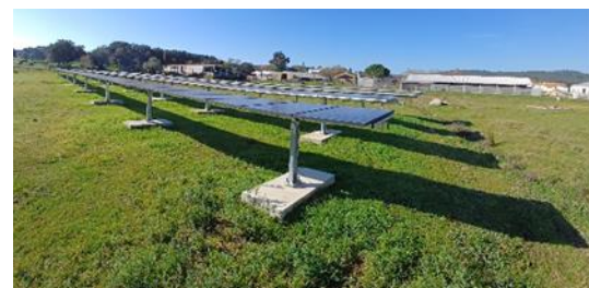
Figure 3: Solar PV Plant
