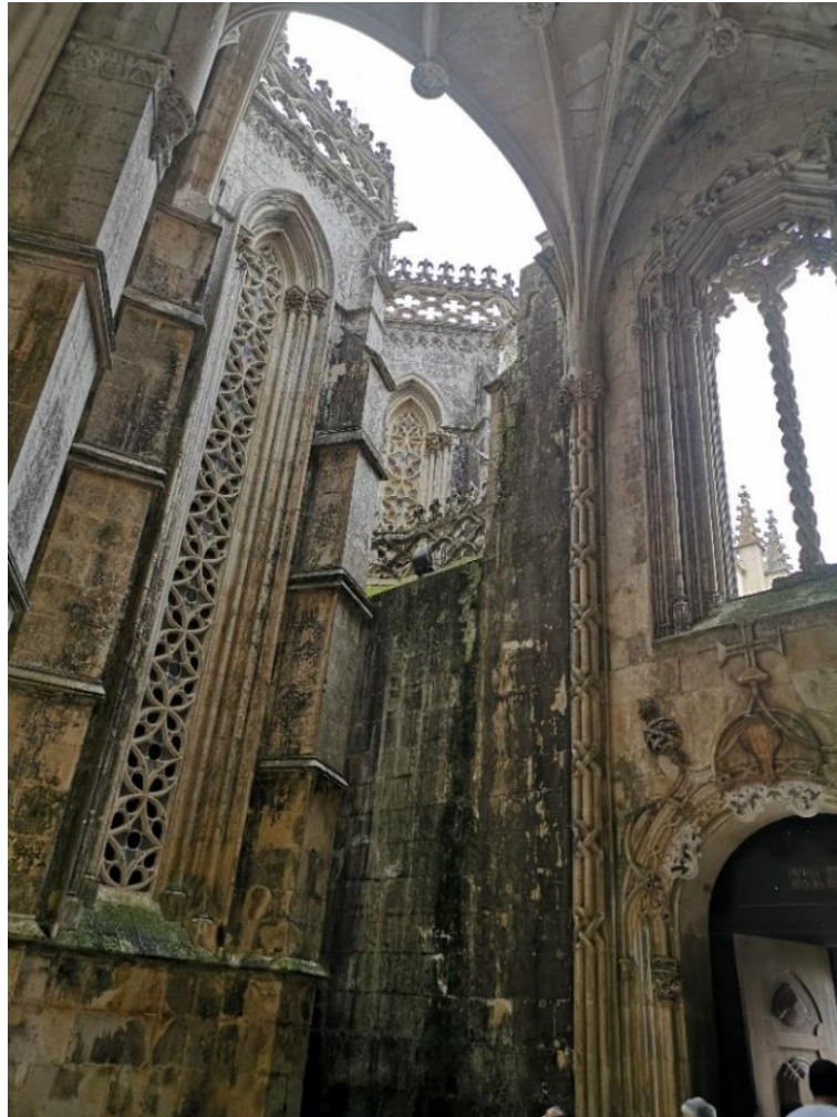
Figure 4.1. Bio-degradation on the inner wall of the “imperfect chapels” of the Batalha Monastery.
