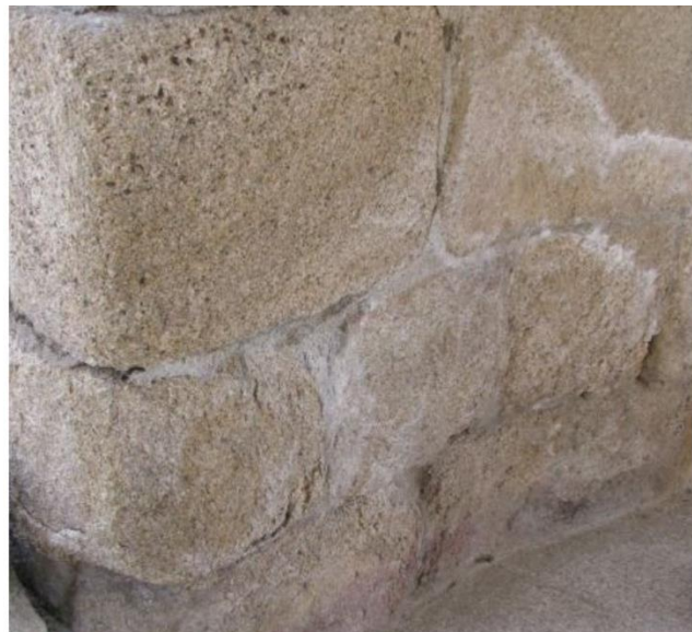
Figure 1.2 Salt efflorescence (the whitish powder) on granitic stones of a window from a historical structure in the town of Chaves, Portugal (Alves, C., et al., 2021).
