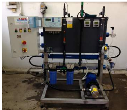
Figure 1. Reverse Osmosis desalination unit
