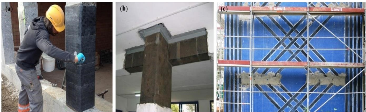
Figure 2. Examples of seismic strengthening with CFRP systems: (a) Jacketing of column, (b) Confinement of beam-column joint (c) Strengthening of concrete wall ( S&P Clever Reinforcement ).
