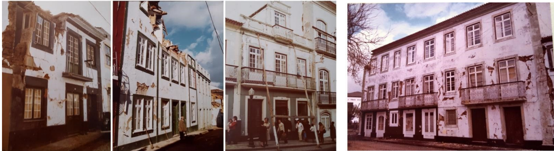
Figure 1. Damage in Angra do Heroísmo, Azores, due to the 1980 earthquake. Example of local mechanisms (left) and of damage in the piers (right) (DGPU, 1980).
