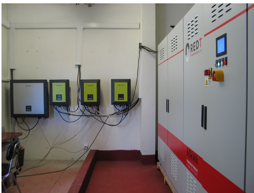
Figure 5.3: VRFB (right) and the inverters (left)
