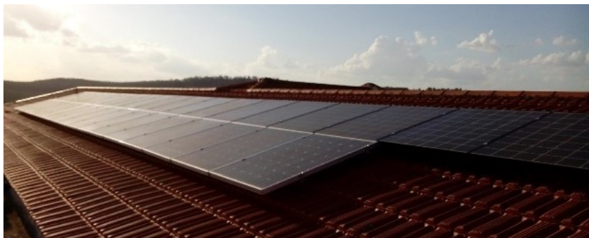
Figure 5.2: Roof mounted PV system
