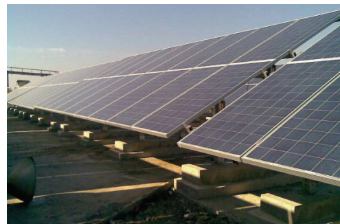
Figure 3: Grid-connected PV installation without shading between consecutive rows.
