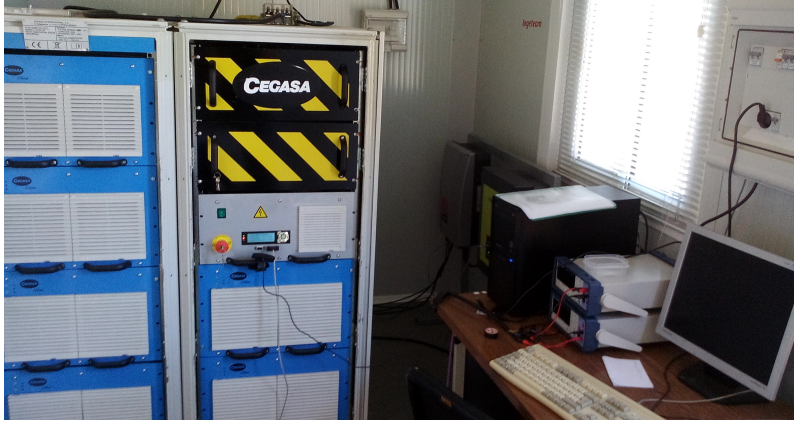
Figure 4.12: Photograph of the LIB prototype system. The battery has a total 32kWh (5.3kWh per blue drawer), and 5kW nominal power.
