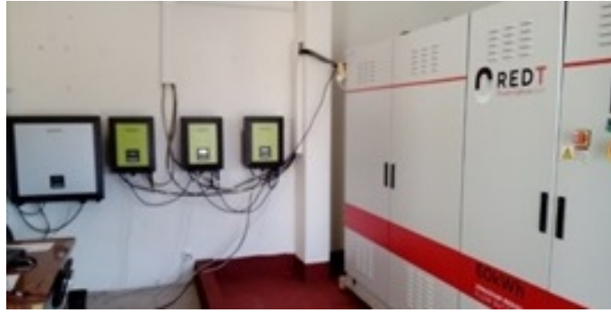
Figure 4.8: Photograph of the site after the prototype system installation: PV and battery power inverters fixed on the wall (in the middle), acid-resistant coated bund (red area in the floor), and the VRFB (inside metal cabinet).
