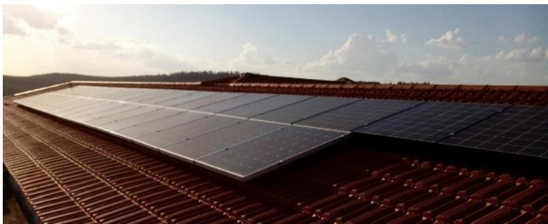
Figure 4.3: Photograph of the BIPV system, mounted in the rooftop near the VRFB prototype site
