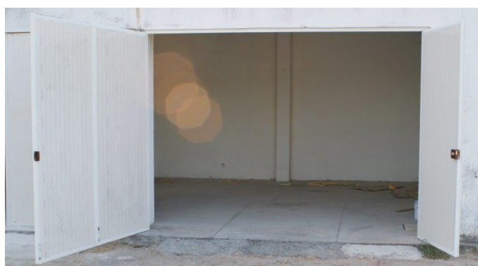
Figure 4.7: Photograph of the porch chosen for the VRFB prototype system, already with walls and doors. This site was designed to have ground access and allowed for easy assembly of the VRFB access for the required machinery.
