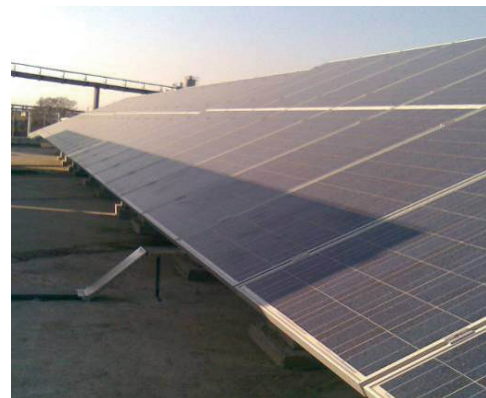
Figure 2: Grid-connected PV installation with a supporting structure that cast a shadow over the panels behind it.
