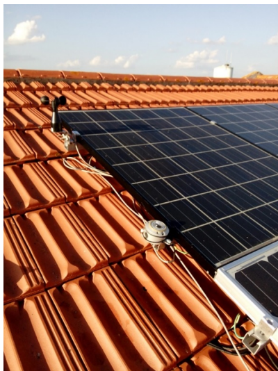
Figure 5.5: Pyranometer and anemometer installed on the roof.
