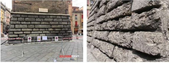
Fig. 10. Degradation of the selenite of the Garisenda tower.
