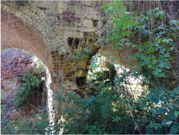
Fig. 7. The heavily damaged pillar.
