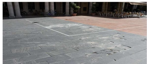
Fig. 2. The typical alteration of stone paving, with the filling of the joints deteriorating and crumbling: this is how the disruption of the entire paving package is triggered.
