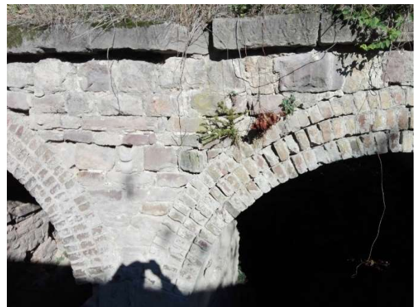
Fig. 6. Degradation of the joints.
