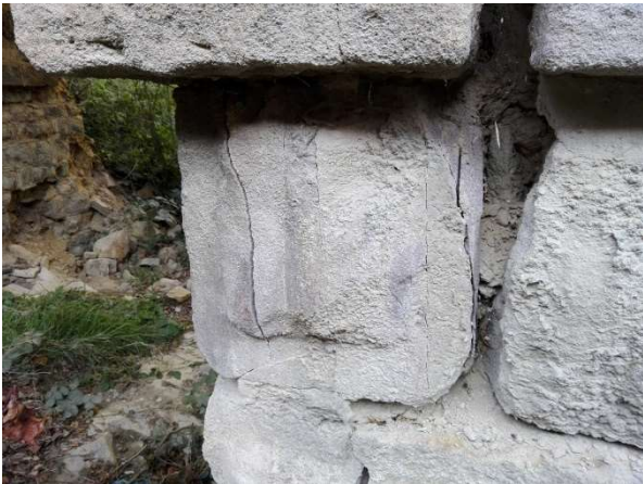
Fig. 8. The cracked sandstone on the corner of a pillar.
