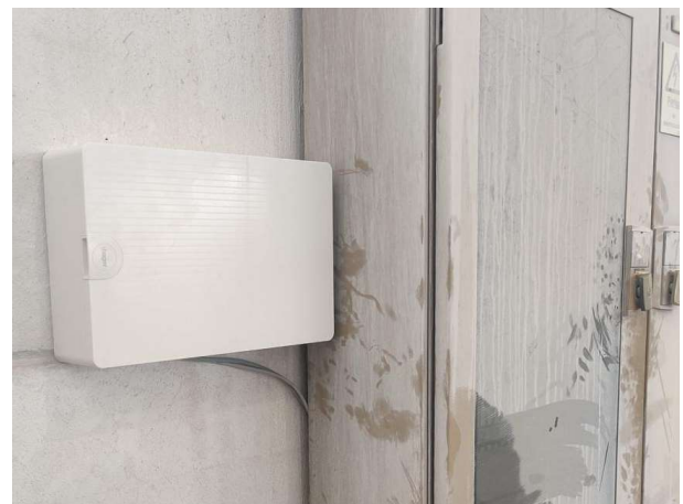
Fig. 1. External switchboard with energy monitoring device.
