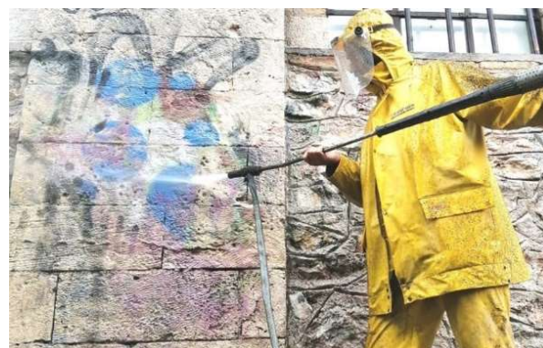
Figure 3- Operation to remove graffiti from Stone buildings using low-pressure water and detergent or solvent.
