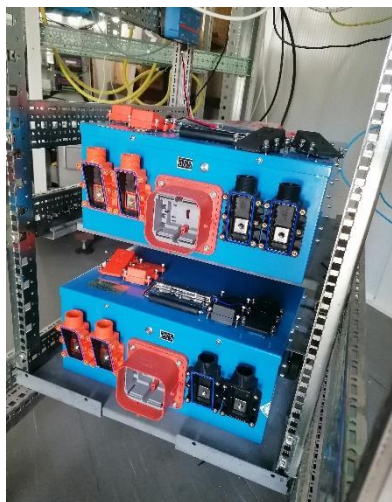
Figure 3: HSupercap installed at CERUÉ's from manufacturer Kurt Energy [2].
