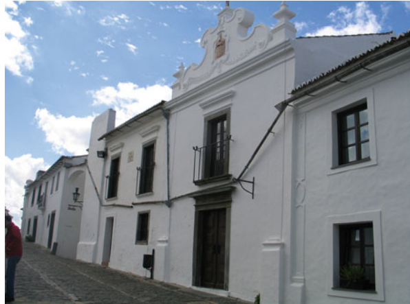
Fig. 4 Rainwater-harvesting system of gutters, placed in the eaves of the house roof in Monsaraz village, Alentejo region, Southern Portugal
