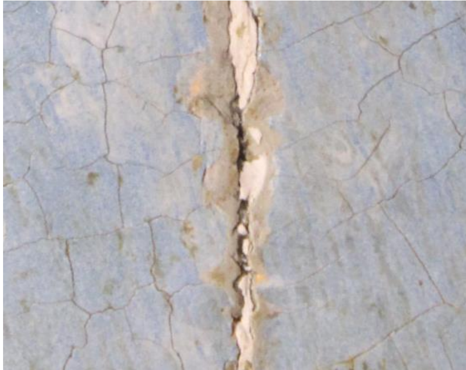
Fig.15. Image showing the pale grey preparation layer exposed along the right crack after cleaning
